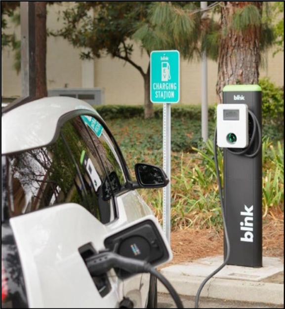
Infrastructure Blink Charging
